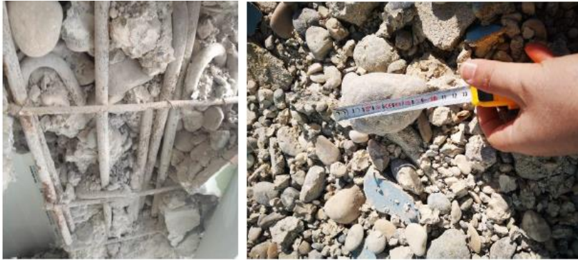
Fig. 14. Poor concrete quality
