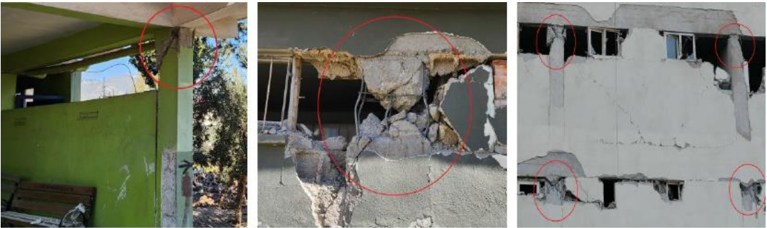
Fig. 7. Structural damage from short column formation
