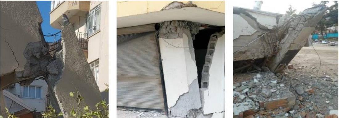
Fig. 8. Column-beam connection failures
