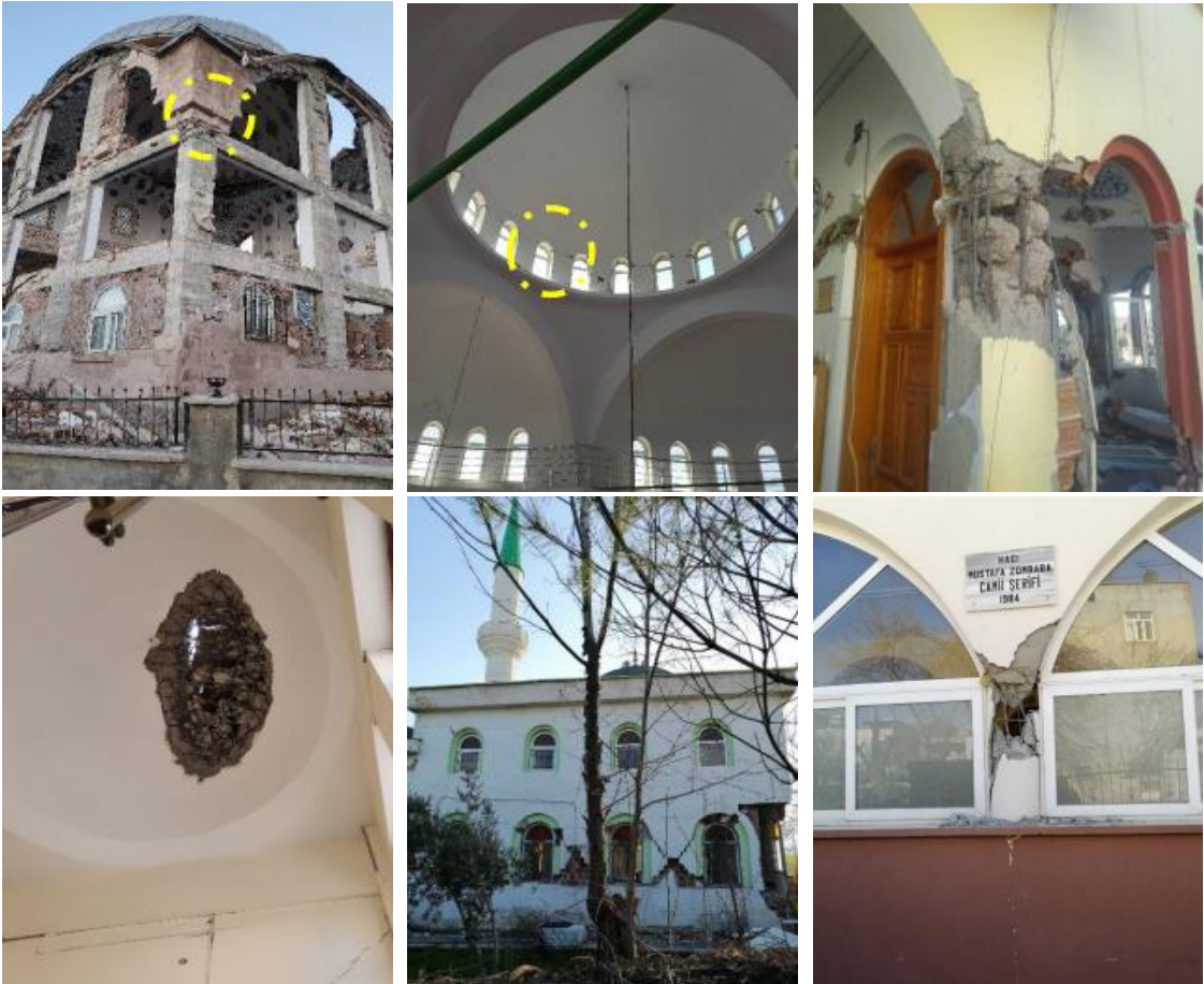
Fig. 25. Observed damages on reinforced concrete mosques
