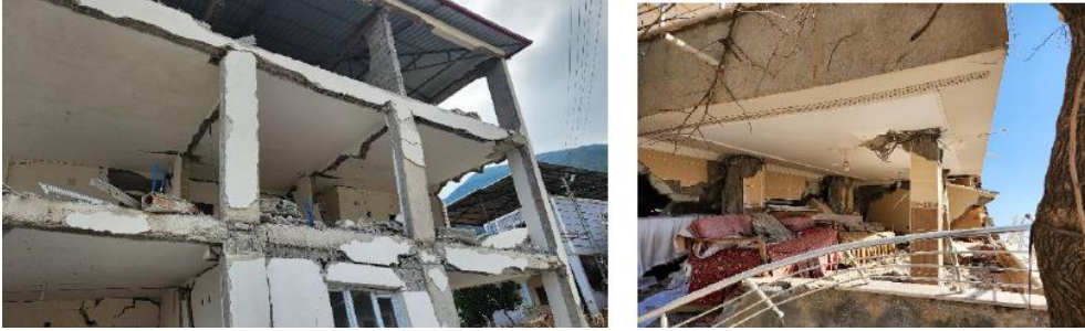
Fig. 12. Damages caused by hollow flooring application
