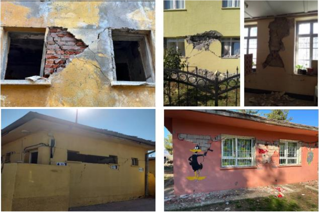
Fig. 17. In-plane damages on masonry buildings
