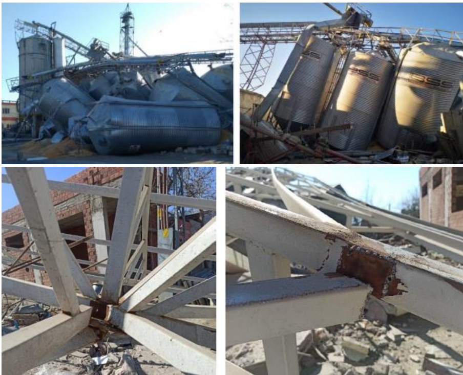
Fig. 19. The damages on steel industrial structures
