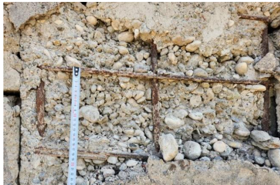
Fig. 15. Unribbed reinforcing bar and corrosion
