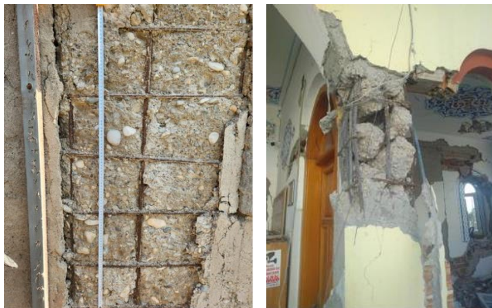
Fig. 11. Insufficient transverse reinforcement
