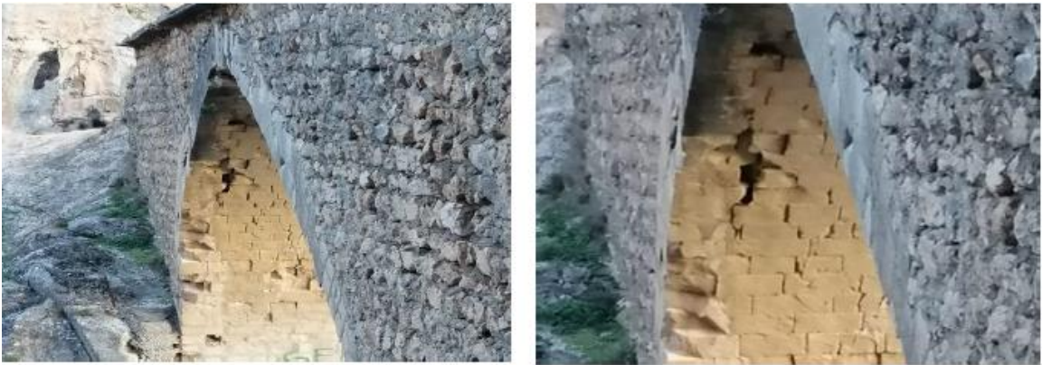
Fig. 23. Damages observed on Devil (Memluk) Bridge
