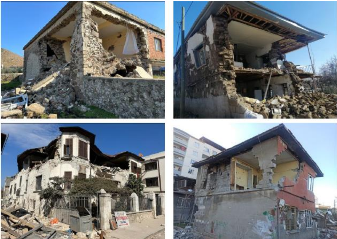
Fig. 18. Out-plane damages on masonry buildings
