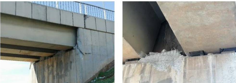
Fig. 22. The joint and support damages
