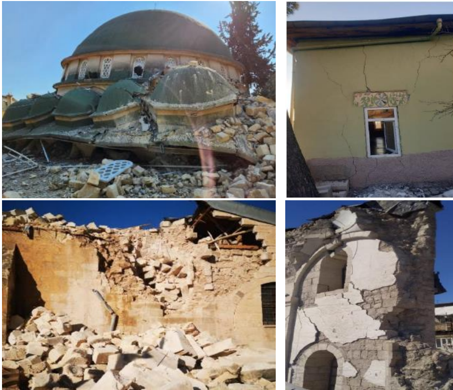
Fig. 26. Observed damages on masonry mosques
