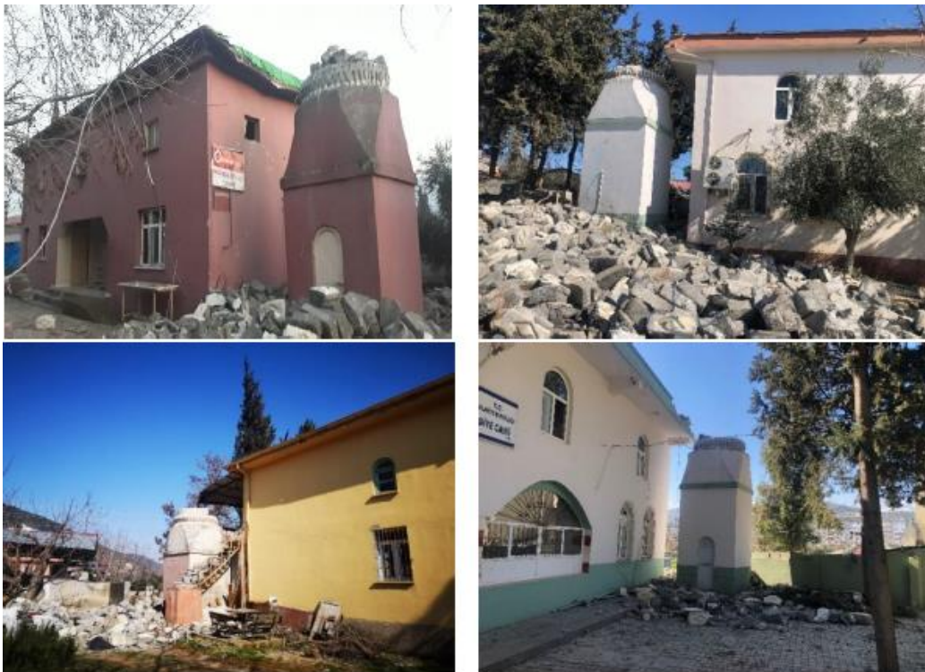
Fig. 28. Observed damages on reinforced masonry minarets
