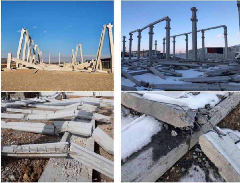
Fig. 20. The damages on steel industrial structures
