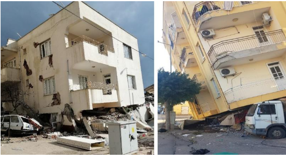
Fig. 13. Soft story damages
