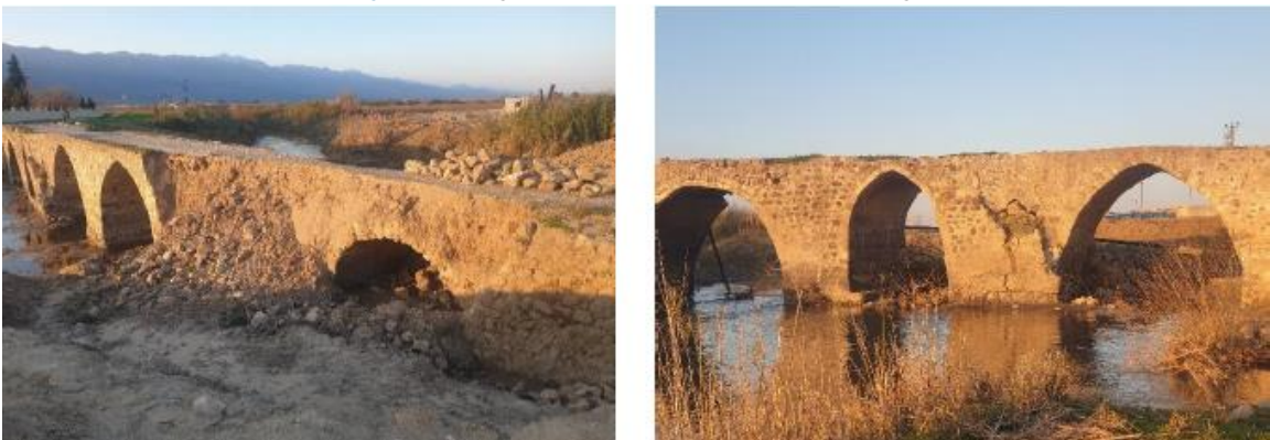
Fig. 24. Observed collapsed and cracks of the spandrel wall
