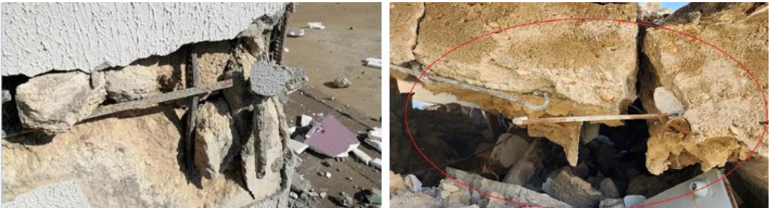
Fig. 9. Existence of short and unconfined lap splices
