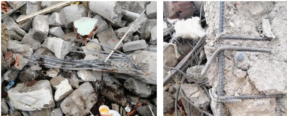
The incorrect placing of the reinforcement bar
