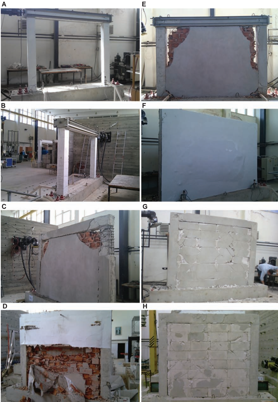
Figure 16: Failure patterns of the test frames. (A) PRCF-1, (B) PRCF-2, (C) RCF-1, (D) RCF-2, (E) RCF-3, (F) RCF-4, (G) RCF-5, (H) RCF-6.
