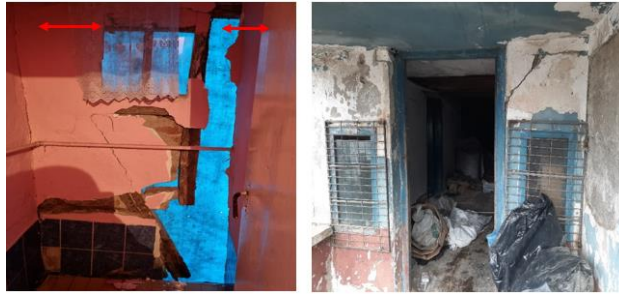
Fig. 26. Damages caused by unsuitable door and window openings
