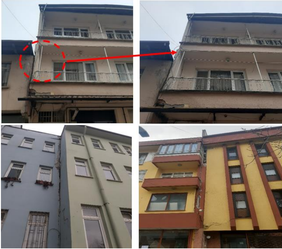
Fig. 14. Damages caused by the inadequate safe distance between adjacent buildings
