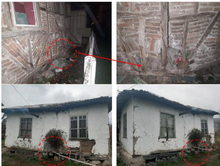
Fig. 31. Damages caused by foundation movement
