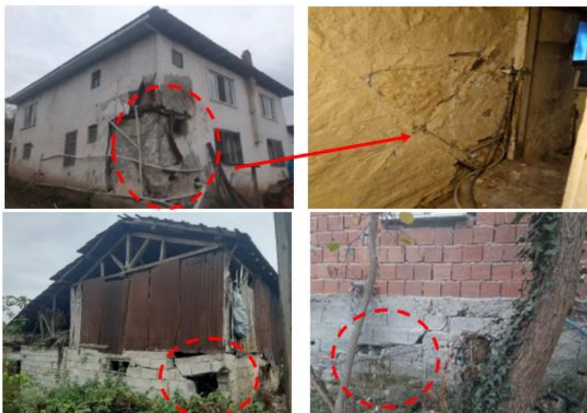
Fig. 28. Vertical crack damage in low-strength masonry units
