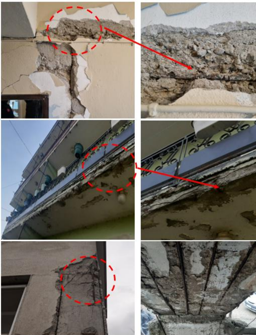
Fig. 21. Damages caused by corroded and unribbed reinforcement steels
