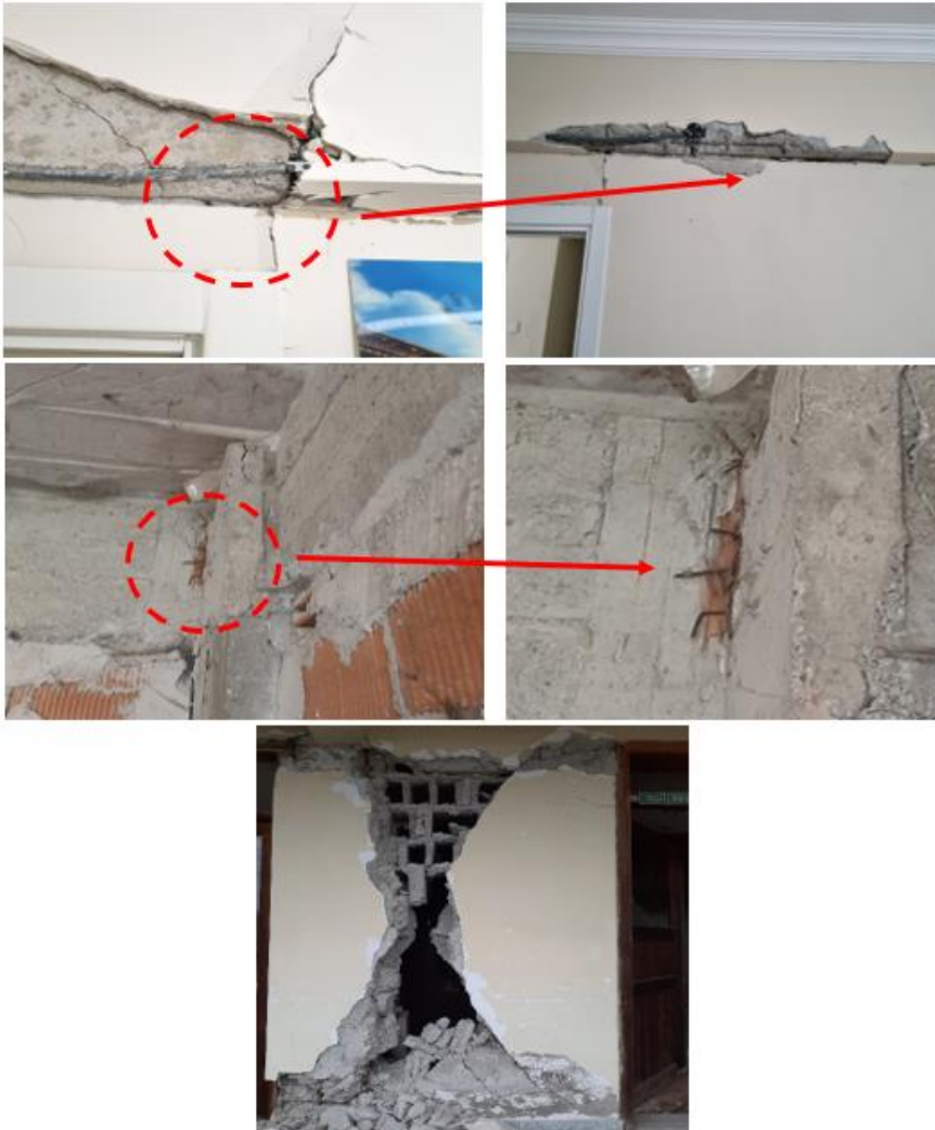
Fig. 22. Damages caused by workmanship defects
