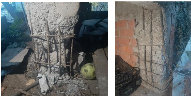
Fig. 16. Observed damages due to insufficient lap splice
