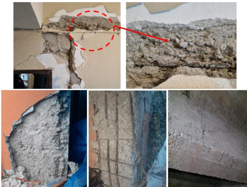
Fig. 23. Damages caused by poor concrete quality
