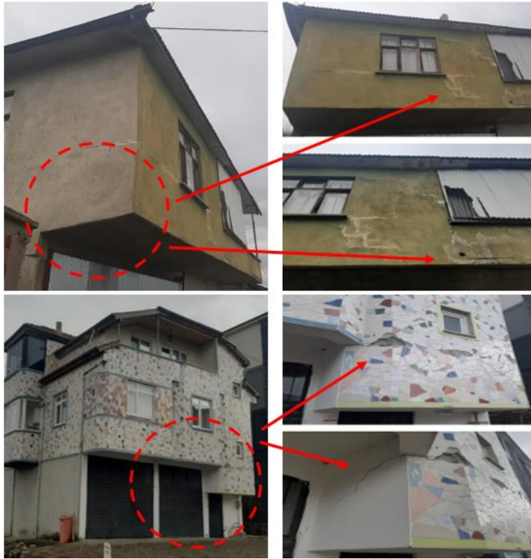
Fig. 17. Damages caused by the long and heavy cantilevers
