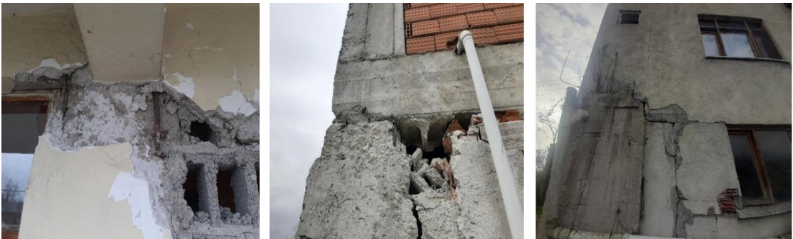
Fig. 15. Damages caused by column-beam connection failures
