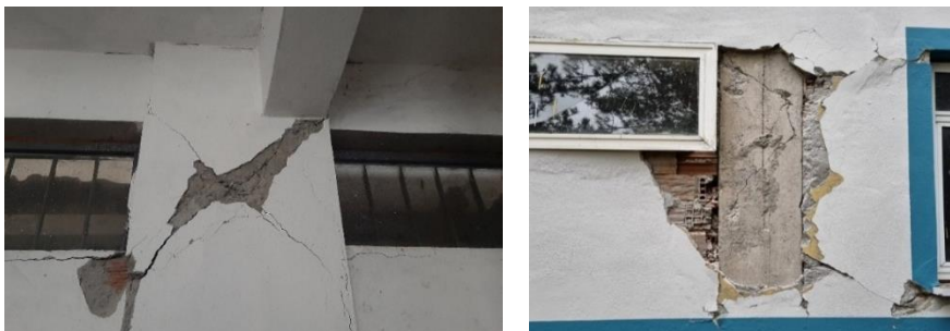
Fig. 13. Damages caused by short column
