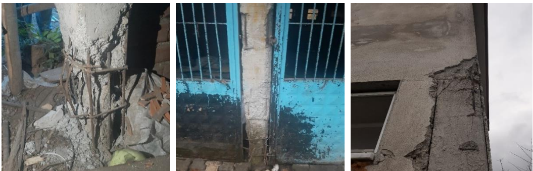
Fig. 20. Damages caused by insufficient transverse reinforcement
