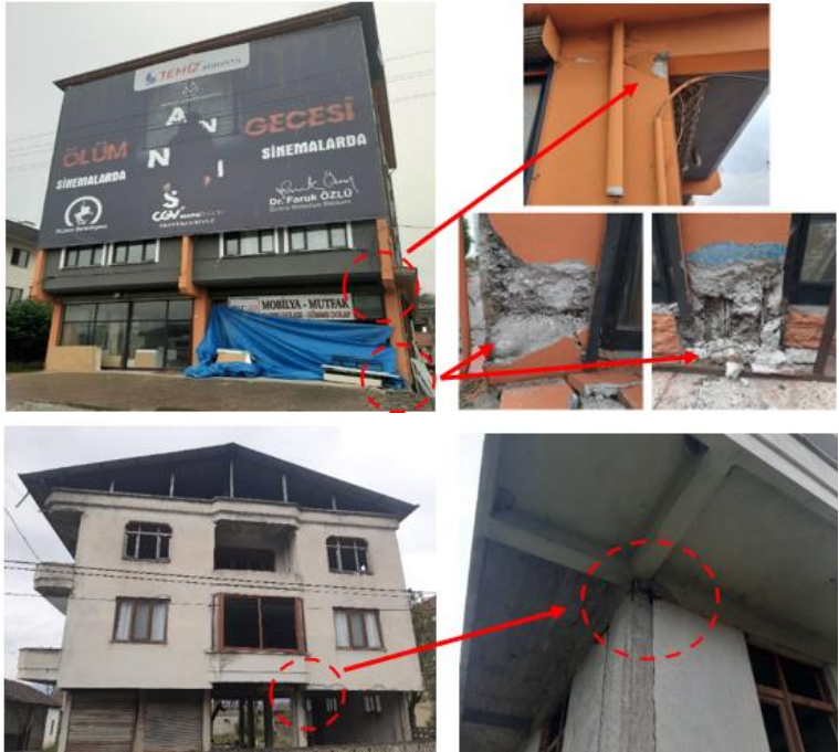
Fig. 18. Damages caused by the soft story
