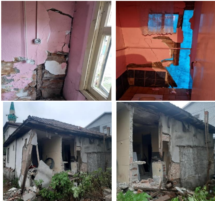
Fig. 25. Damages caused by unsuitable connection details of the vertical walls
