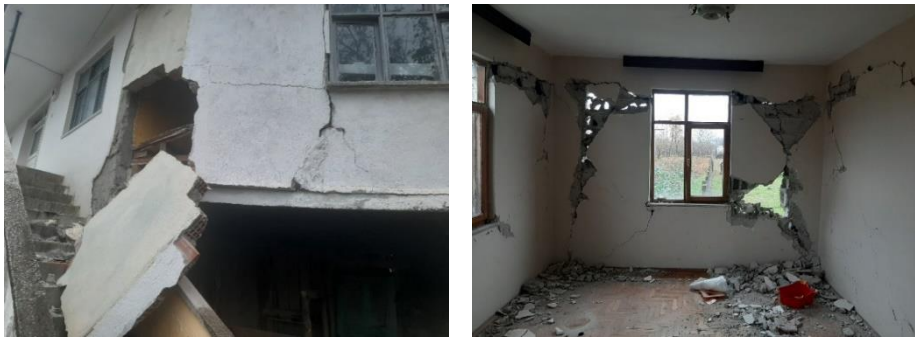
Fig. 19. Weak infill wall damages
