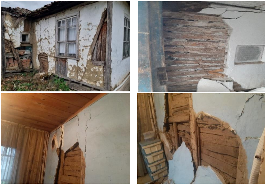
Fig. 27. Vertical crack damage in low-strength adobe units
