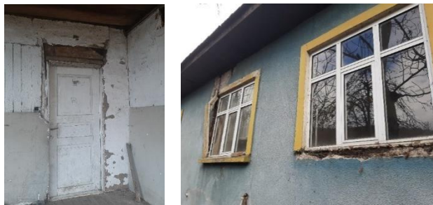
Fig. 30. Damage occurred due to insufficient lintel length
