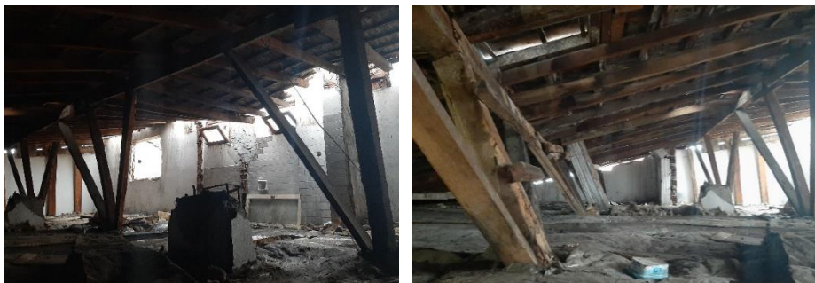
Fig. 24. Damages caused by the weak gable wall
